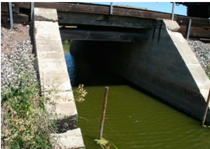
This UPRR bridge will be replaced as part of an effort to improve the wildlife habitat in McNabney Marsh.
