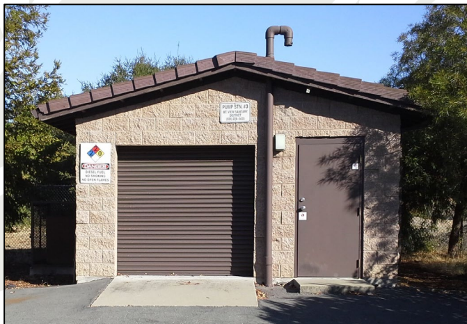
Pump Station No. 3
