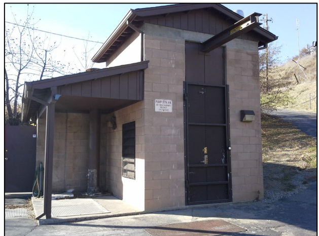
Pump Station No. 4
