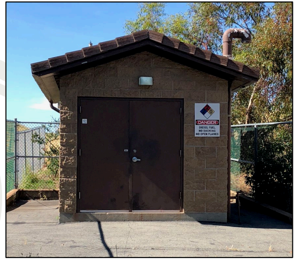
Pump Station No. 2
